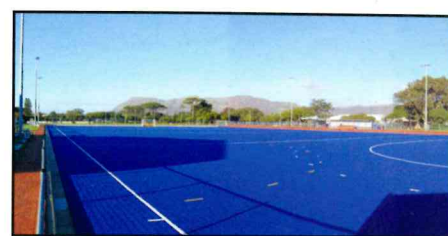
Strata Civils pays particular attention to the tolerances on the final surface of the turf, which is critical to the quality of the final playing surface
